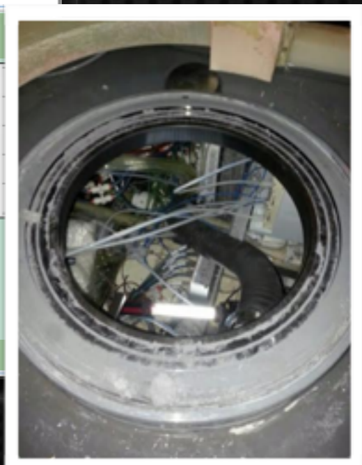
Rusty bearings caused the unstable torque, which incurred abnormal vibration
